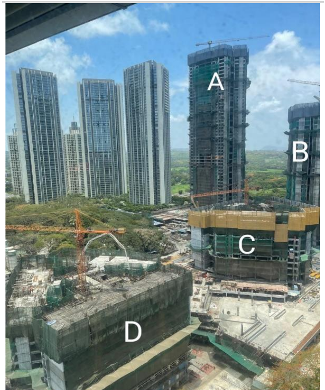
Exhibit 8: OBER – Work on Tower D (likely under launch planning) of Elysian already commenced
